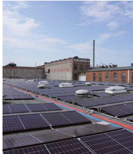
Developing renewable energy By the end of 2024, we have deployed 68,500m 2 of photovoltaic panels on 5 of our industrial and logistics sites around the world. We will continue these efforts to achieve 50% decarbonised energy in our energy mix by 2025.
